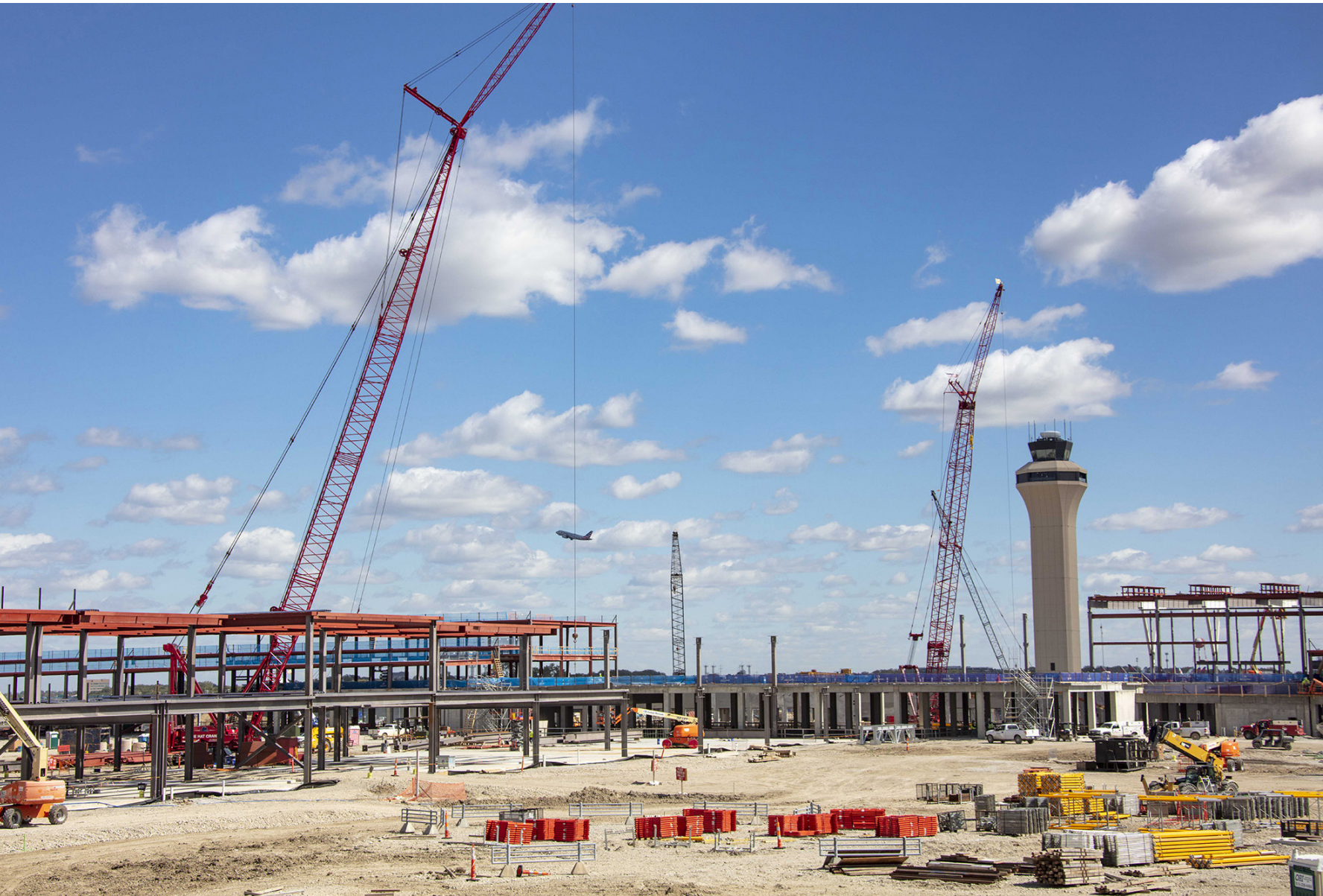
In this photo from October 2020, crews erect structural steel at the New Terminal while flights depart and arrive at the existing terminal in the distance. Photo by: From the Ground Up Photography
