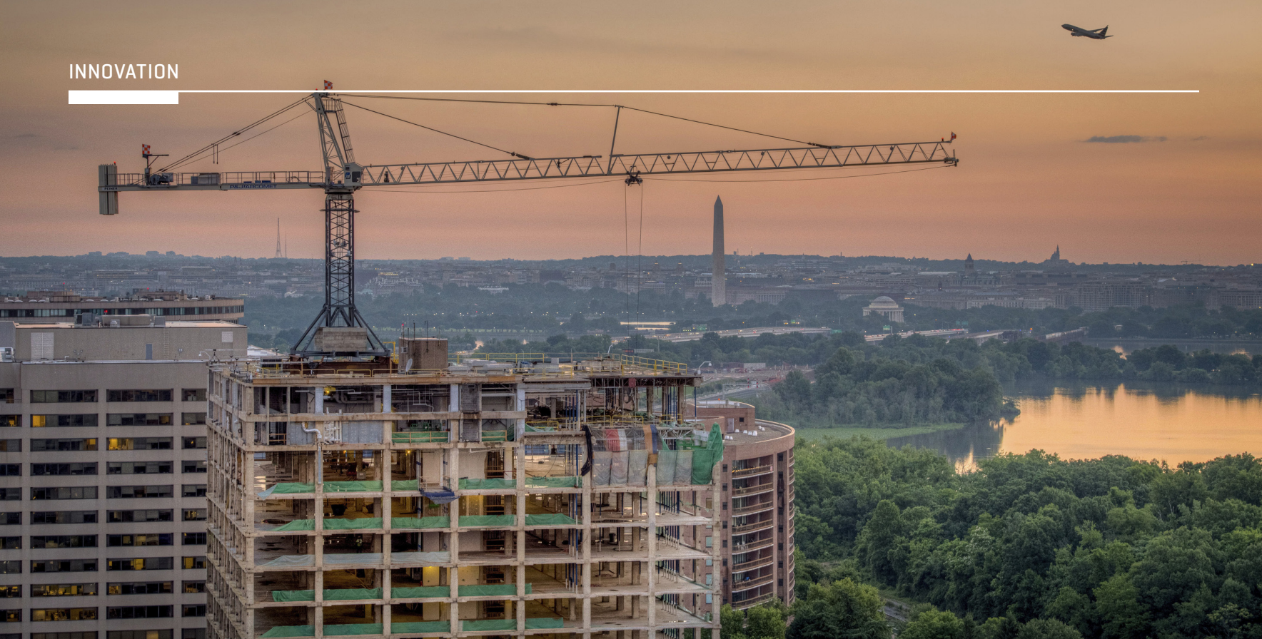
A roof-mounted crane used at 1770 Crystal Drive has helped the project team navigate challenging site logistics.
