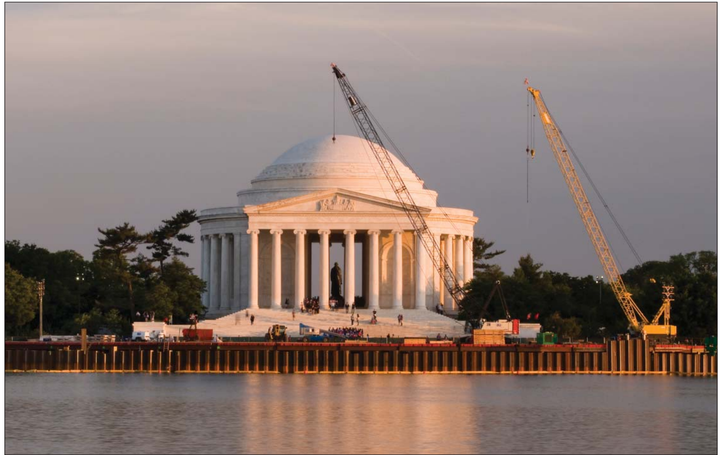
Work is underway on the Jefferson Memorial Seawall, Washington, D.C. (Photo by Dan Cunningham)
