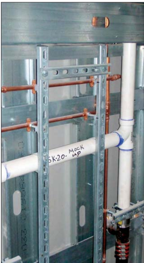
Each of the NCB's operating rooms has up to 16 medical gas lines. In-wall system mock-ups ensured that each line worked properly and was without obstruction.
