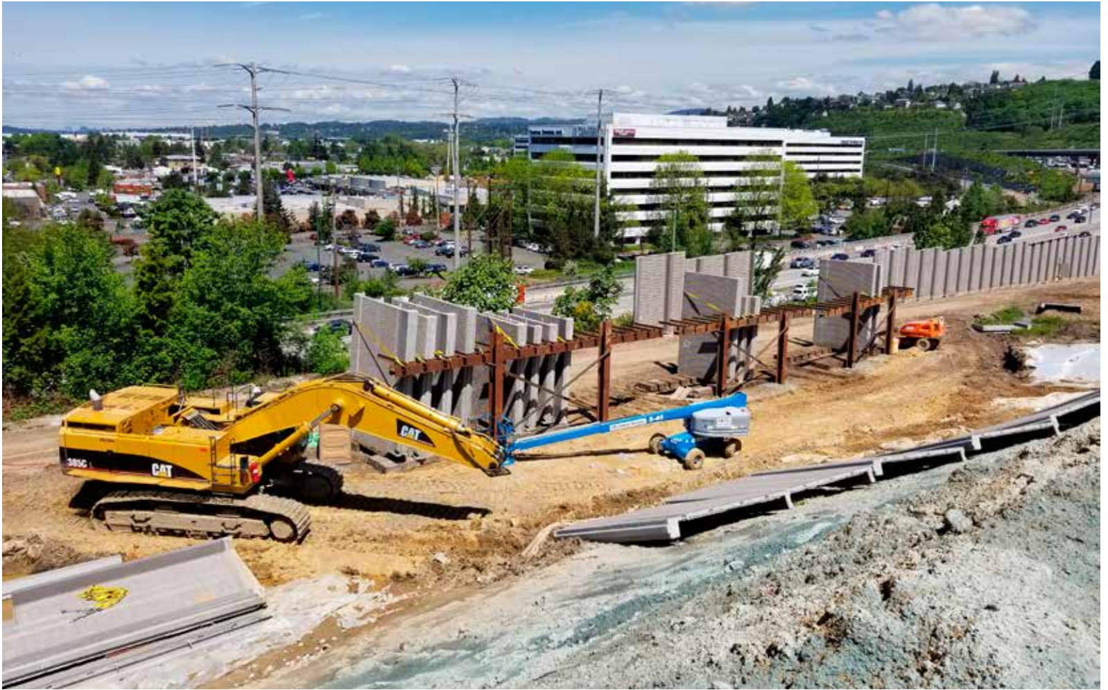
The sound barrier panels were removed and stored on a custom storage rack until they were ready for placement.
