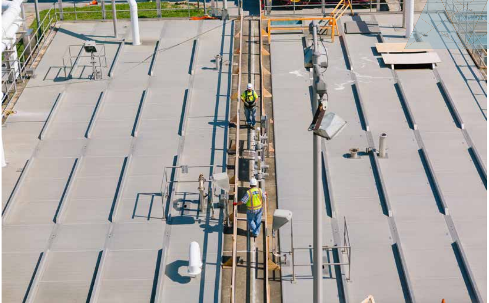
This page: Temporary handrails are inspected before removing tank covers at the Little Patuxent Water Reclamation Plant.
