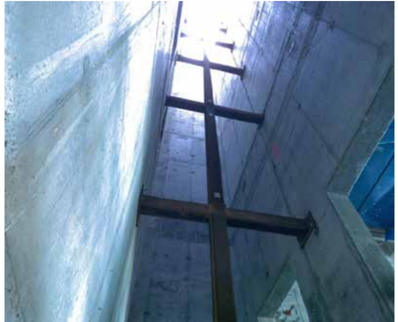
On the Miami Beach Convention Center project, the Field Engineering Group verified elevator hoistway geometry using 3D laser scanning.
