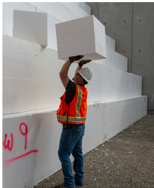
Above: Atkinson's team used a solution for the ramp that was as light as a feather—or, more accurately, as light as 700,000 pounds. The team used 2,700 geofoam blocks to replace soft underlying soil. Each standard block weighs 248 pounds.
